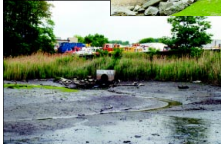
The contaminants that are generated on land find their way to bays, beaches and harbors through storm water outfall pipes like this one, pictured upper right. Outfalls tend to be hidden but the contaminants they discharge result in serious impacts to our special places along the coast. Photos courtesy of Eileen Keenan
