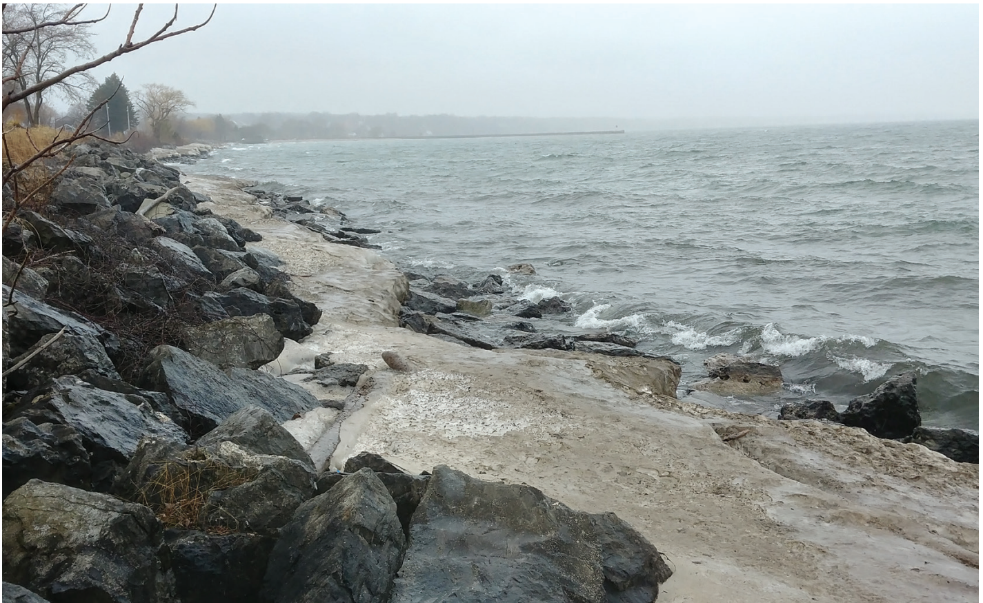
Ice-covered rock rip-rap revetment, Irondequoit Bay (Monroe County, NY). Photo by Roy Widrig, New York Sea Grant.
