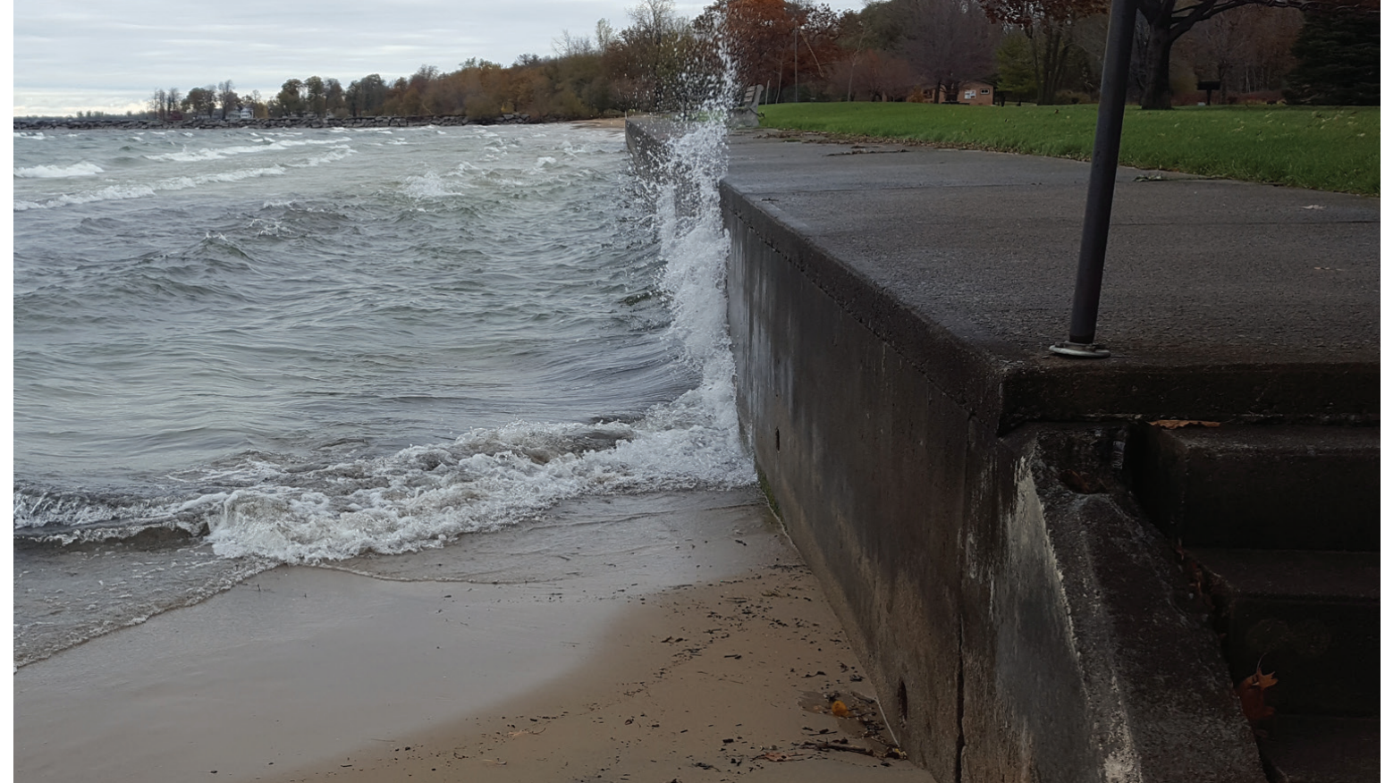
Concrete bulkhead deflecting waves, Westcott Beach State Park. Photo by Roy Widrig, New York Sea Grant.
