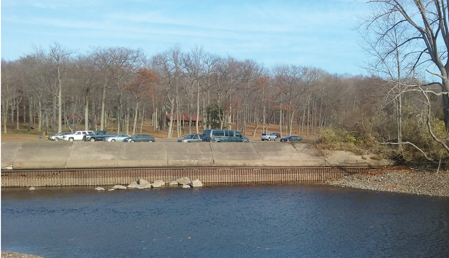
Concrete and steel sheet pile seawall protecting a small harbor, Selkirk Shores State Park (Jefferson County, NY). Photo by Emily Sheridan, New York State Department of Environmental Conservation.
